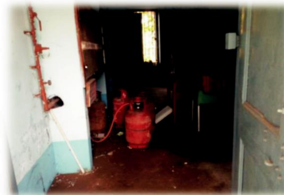
LPG gas use for chemistry lab.
