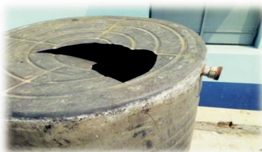
Polluted water in Unusable tank
